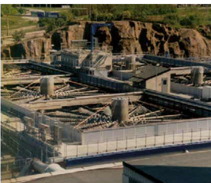
Nitrification Filters, Gothenburg, Sweden
